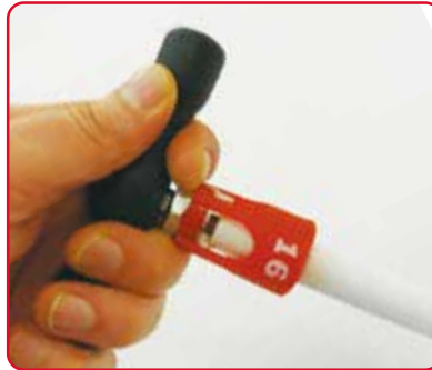
2. Bevel the cut end of the pipe. (applies to MLC Pipes only)
