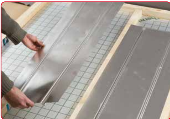
1. Heat emission plates laid between the joists at 400mm centres and secured using suitable fixings.
